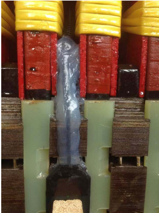
Figure 25a. AGS Sensor probe mounting position showing triax cable and silicone coating
